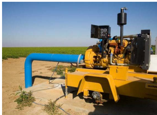
Figure 6.6 Irrigation system pump.
