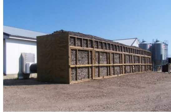
Figure 2.8 A vertical bed biofilter at a University of Minnesota research farm (image courtesy of Iowa State University).
